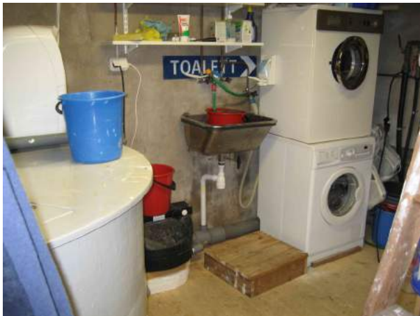
A well maintaind Aquatron doesn't smell and the area of installation can be used for other activitys.
